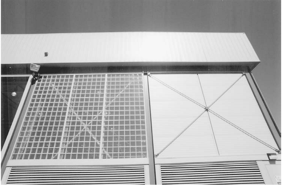
FIGURE 11.10 Presence of glass block in this metal building system justifies strict limits on building drift and racking. Note the interior wall bracing made of steel angles. (The exposed exterior bracing at right is purely cosmetic.) (Photo: Maguire Group Inc.)
